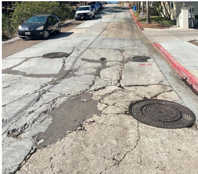
Figure 1: Example of sunken asphalt created by leaking underlying water main.
